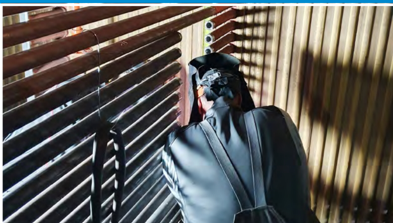
BASF Antwerp GuD power plant in Antwerp Repair of steam boiler July - August 2020
